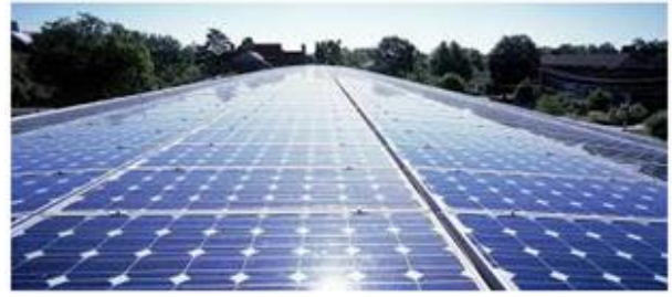
Fig: 3.2 Solar Photovoltaic (PV) Panels
